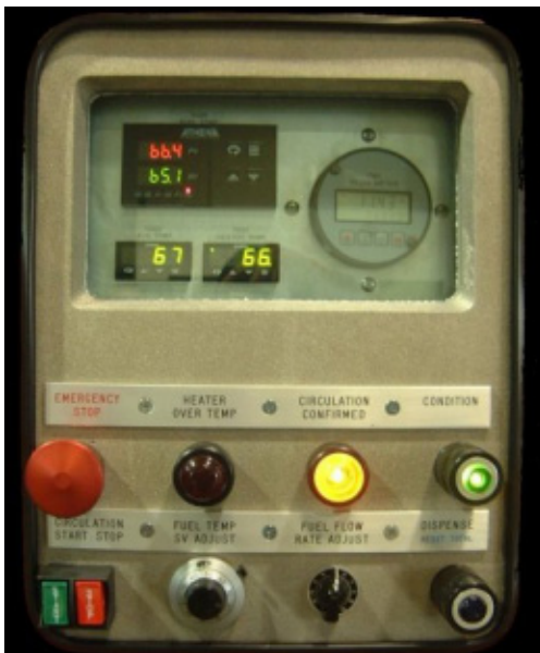
Fuel Conditioning Cart Controls
