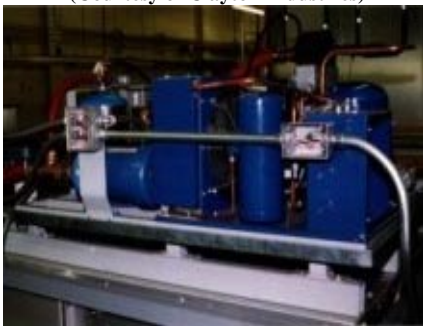
Heating & Cooling Unit
